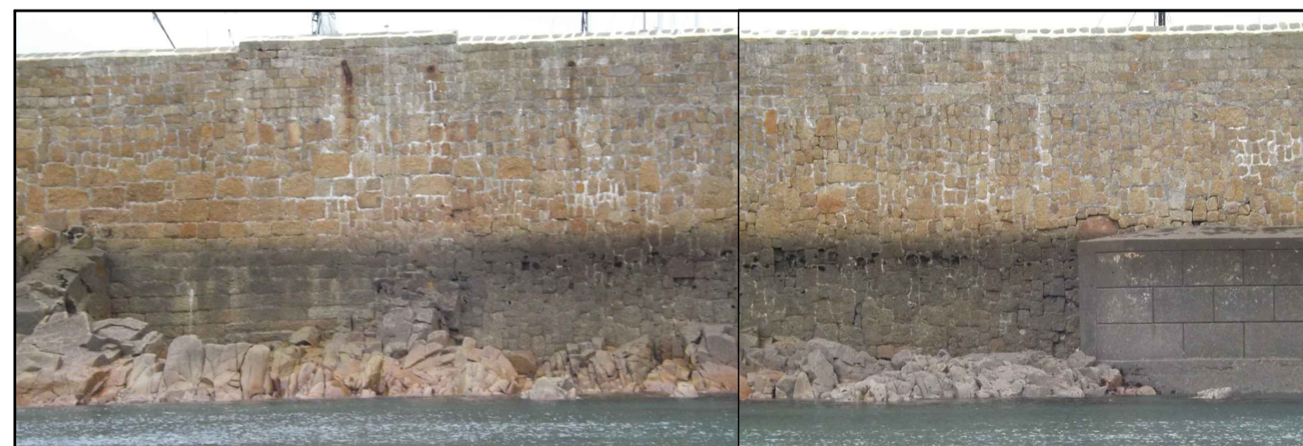
Photo 7 - South Pier - Exposed Area to the Left of Concrete Build-out 2013 RHDHV Inspection
