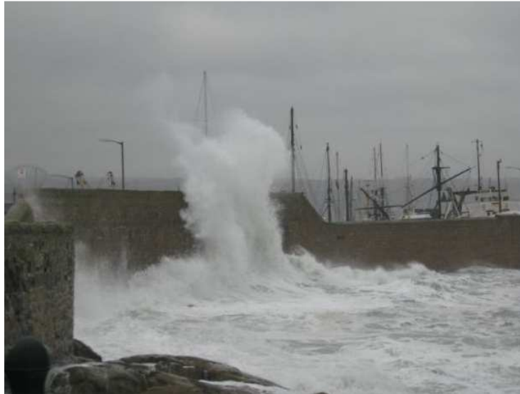
Photo 3 - Wave Overtopping at the Rock Armour in front of South Pier (Courtesy Dave Simpson, Cornwall Council)
