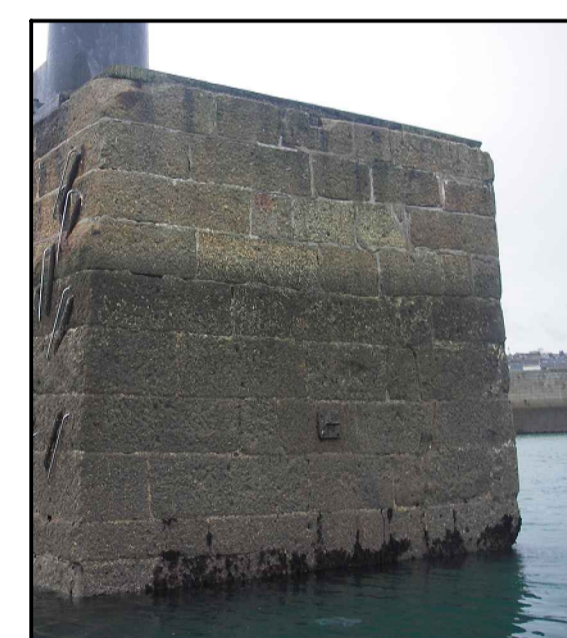
Photo 24 - End Section of Lighthouse Pier 2013 RHDHV Inspection
